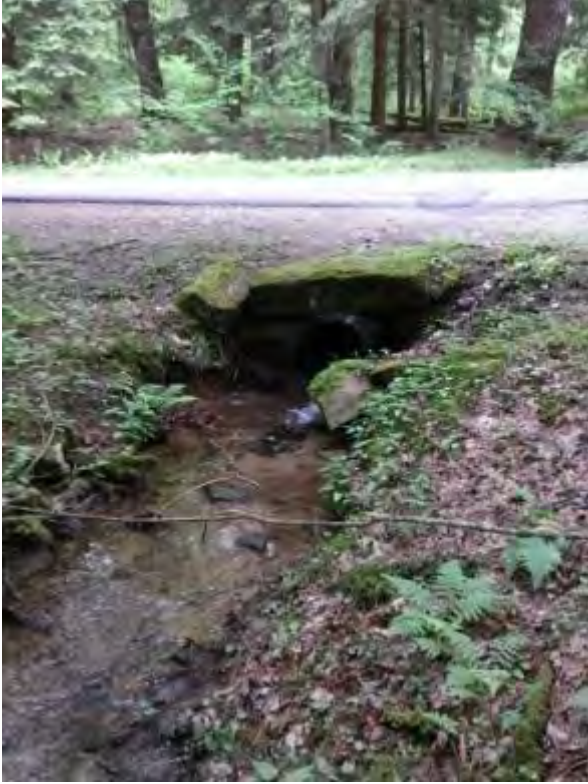
408: Culvert on Clear Creek Park Road is perched and undersized.
