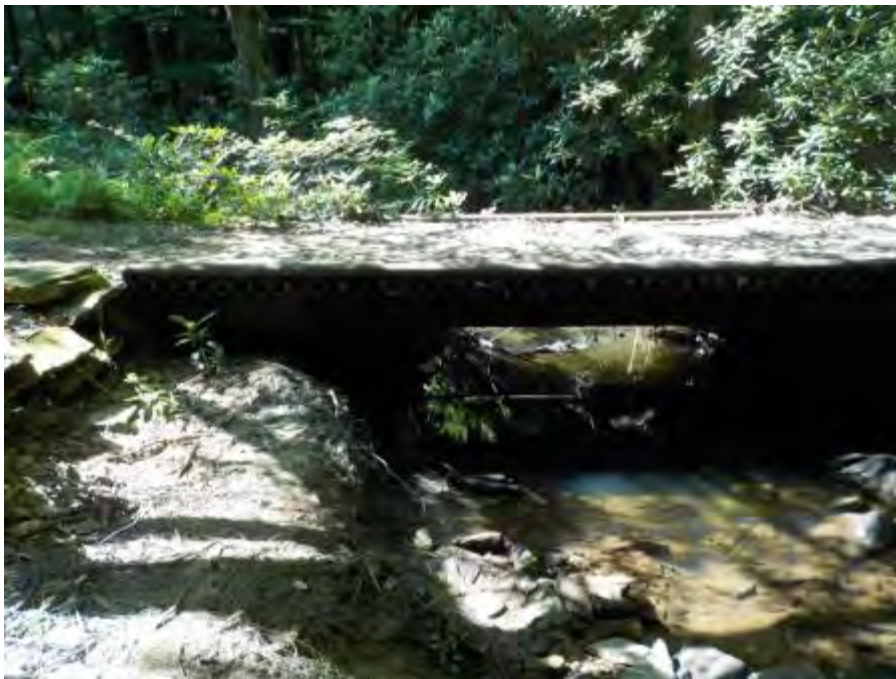
547: While not much of an AOP barrier, this small bridge over Trap Run does constrict the natural stream channel during high flow.
