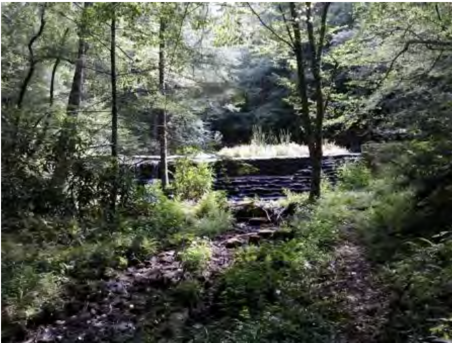
1567: Breastworks (from downstream, a migrating fish's perspective) of the "upper dam" on Callen Run. It is upstream of the bridge where Callen Run Road crosses this segment.
