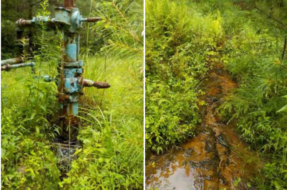
499: A gas well near the top of this segment on the right descending bank leaks discolored, Sulphur-smelling water that is 9.5°C, pH 7.88, and 297 \mu s/cm. The stream does not appear to be mortally impaired from this source, but the water leak is recommended to be plugged in the event that the outflow changes in volume or chemistry.
