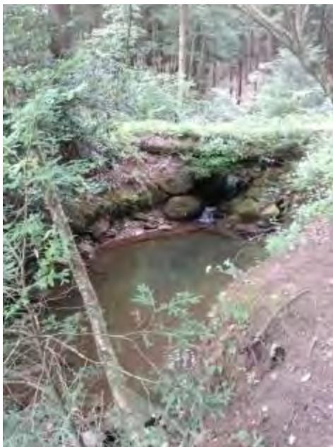
363: A culvert near the mouth of Pine Run is undersized, perched, and has no substrate inside.
