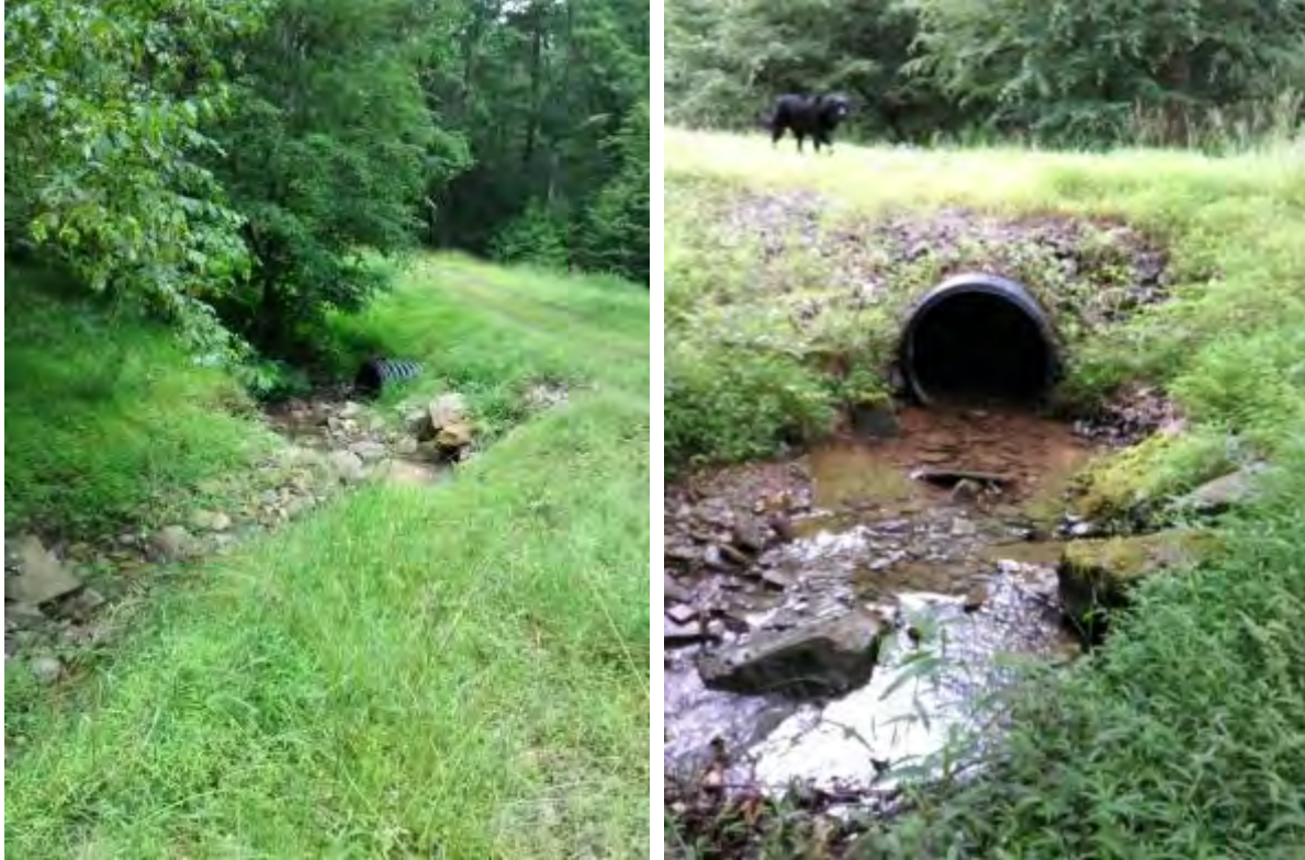
535: Culvert on a State Forest road is undersized and poorly aligned. Inlet with sediment wedge (left) and outlet with scour pool (right).
