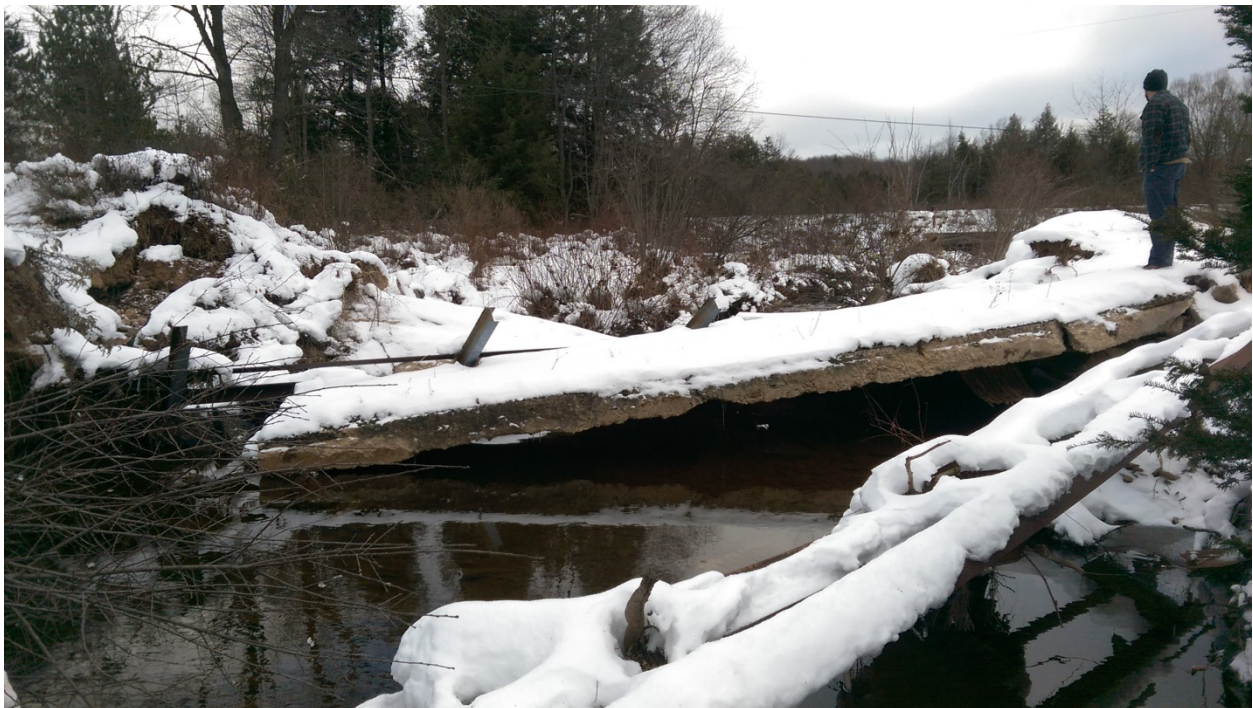
Figure 25. Collapsed road-stream crossing on Old Ellenton Mountain Road following flooding event.
