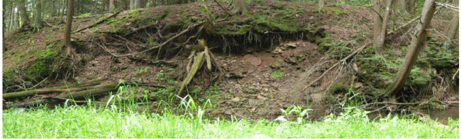
FIGURE 28. Bank erosion on Windfall Run
