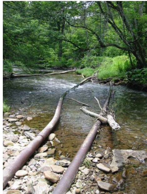
FIGURE 5. Exposed pipelines on Upper Kettle.
