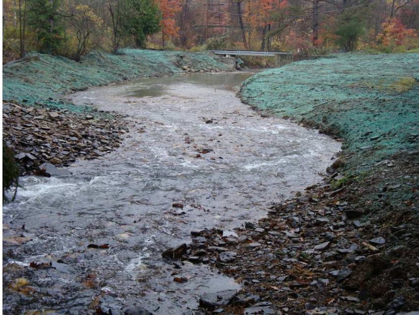
Figure 10: Morrison Run After Lower Dam Removal Removal of the dam was just one of many planned projects on the watershed which contribute to the return to natural flow regimes. Photo credit: Mike Fidale, CCTU
