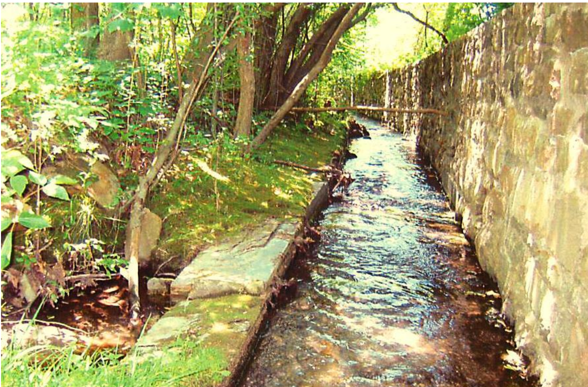
Increased water depths from rain storms are permitted to overflow side bank into remaining buffer area.
