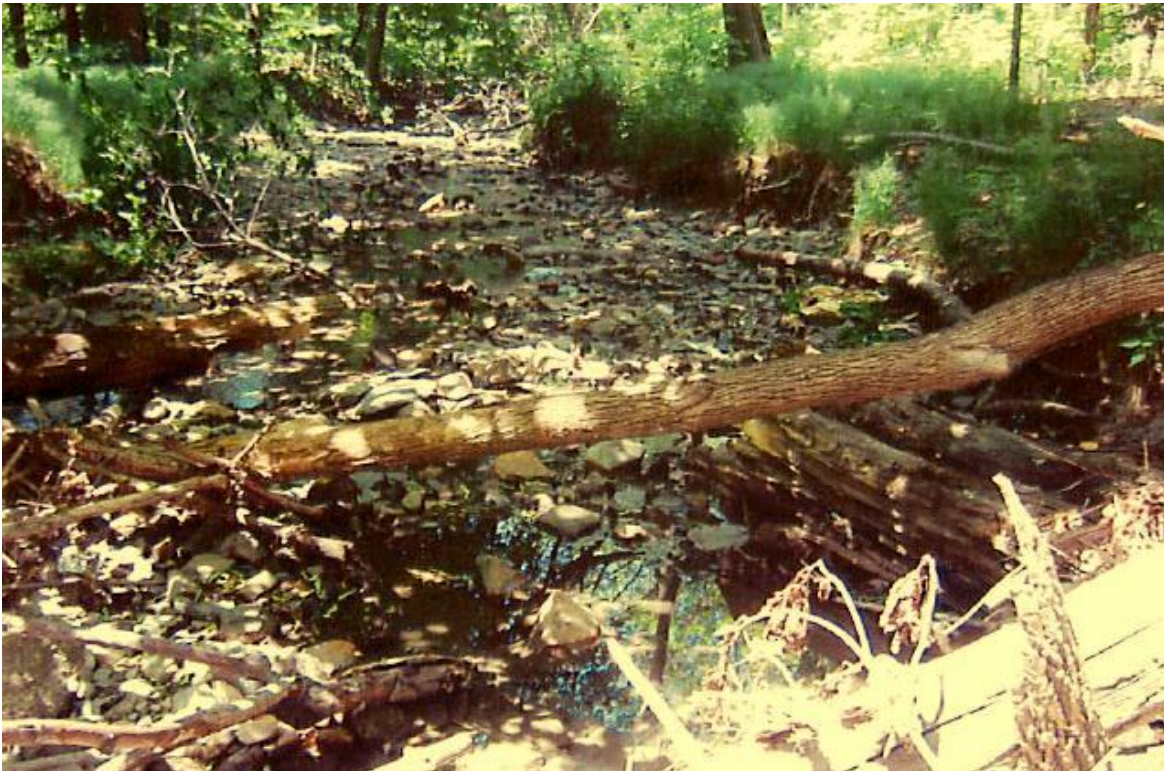
The creek will find the path of least resistance to maintain flow and due to the debris obstructions, the creek has widened
