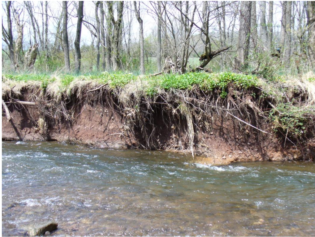
Severe erosion is evident and a major concern.
