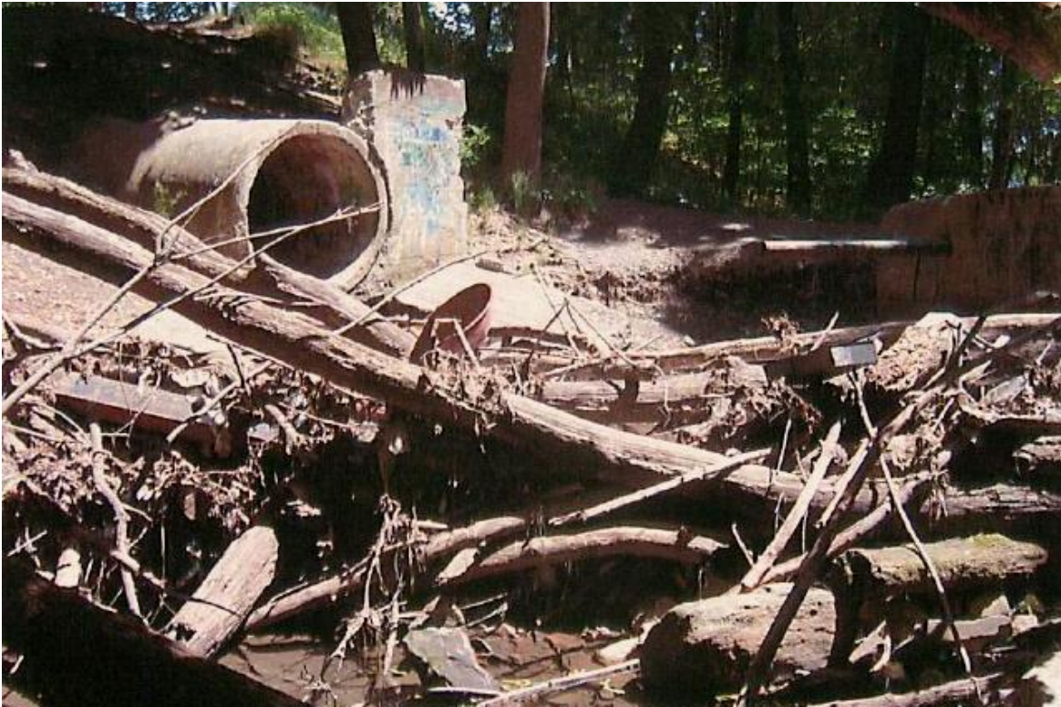
Excessive pile of debris within creek also includes non-biodegradable material harmful to the overall health of creek.
