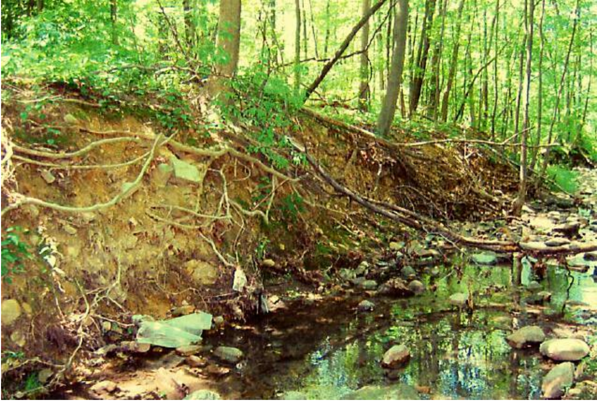
View of severe bank erosion.
