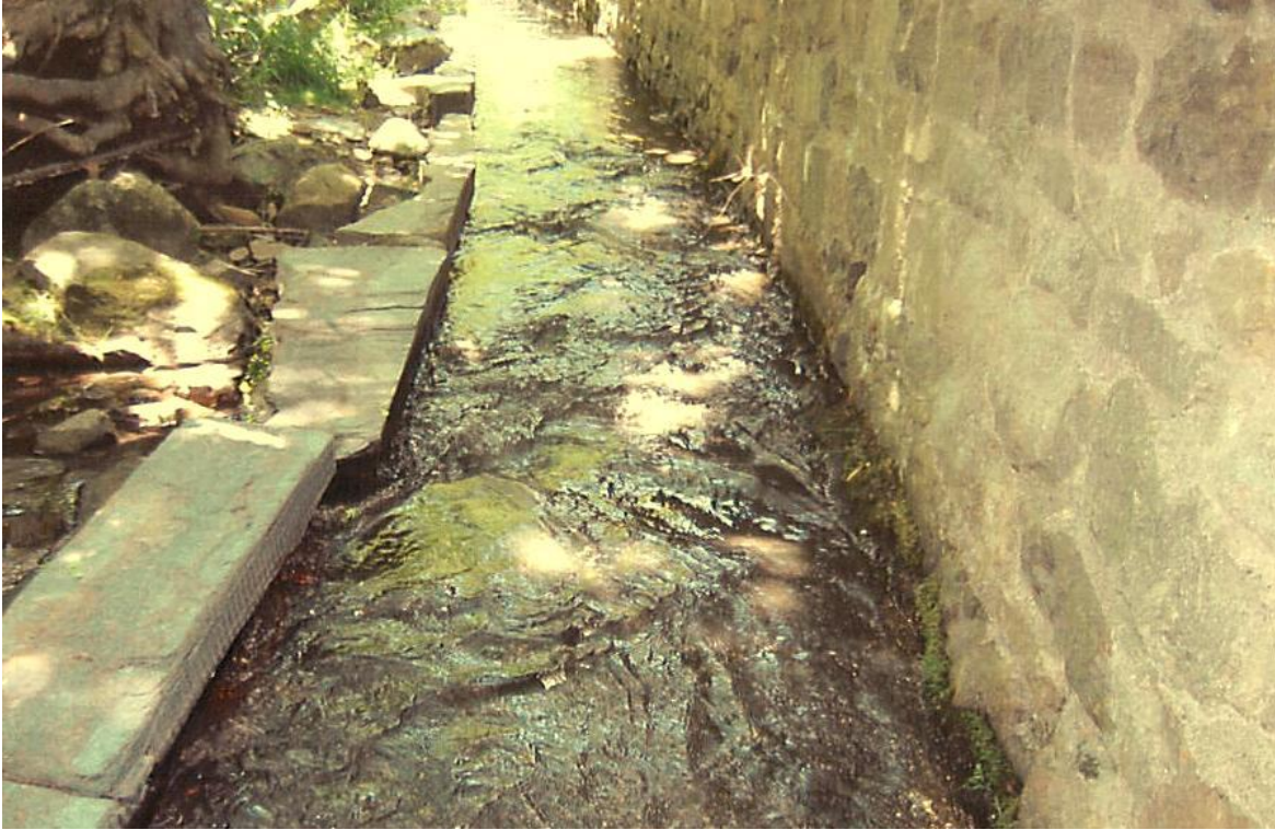
Channeling watercourse will influence overall health of creek, recreational uses and availability of diverse habitats.
