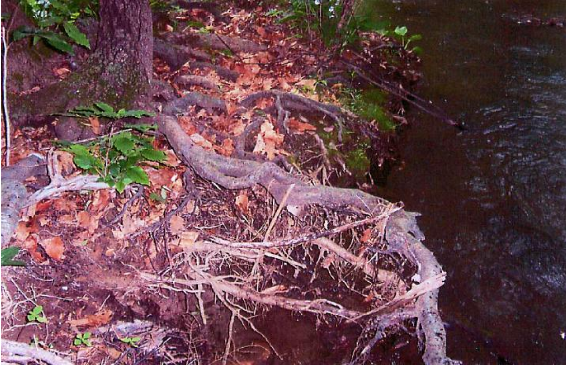
There are areas of exposed tree roots and erosion where banks are not reinforced.
