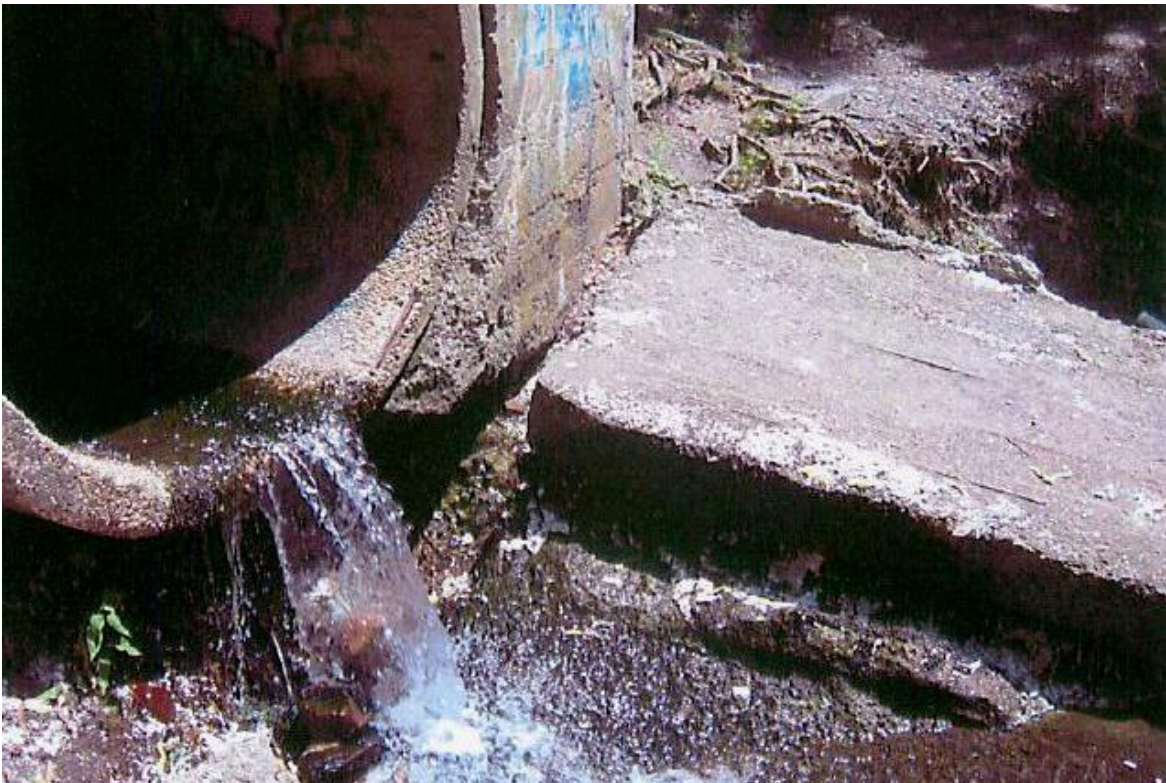
This shows evidence of storm water discharging into creek by nearby quarry.
