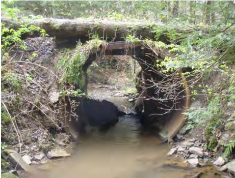
6202: Undersized culvert on private access road.
