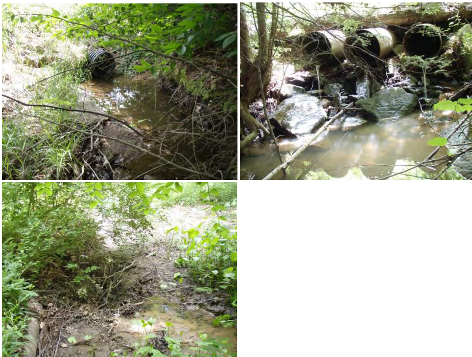
6114: Clockwise from bottom left: Inlet to underground section; outlet of undersized culvert on Pennsylvania Avenue, three undersized pipes on private gas road crossing.
