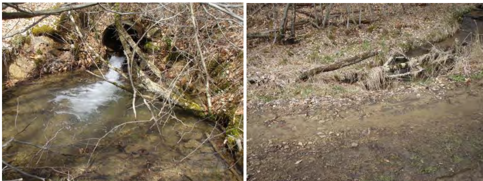
6041: Several undersized/perched culverts for multiple sinuous DGR crossings. Outlet on the left and clogged inlet on the right.
