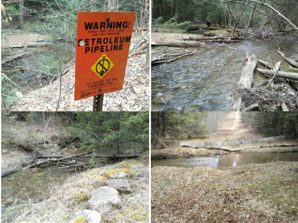
6234: Mobile pieces of wood in the channel may pose risks to exposed infrastructure. Note the absence of larger pieces of wood near these concerns.
