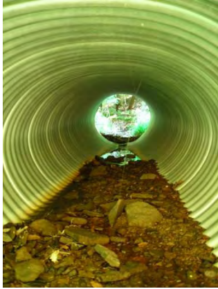
5853: Culvert lacking substrate the entire length of pipe. Note blockage at visible end.
