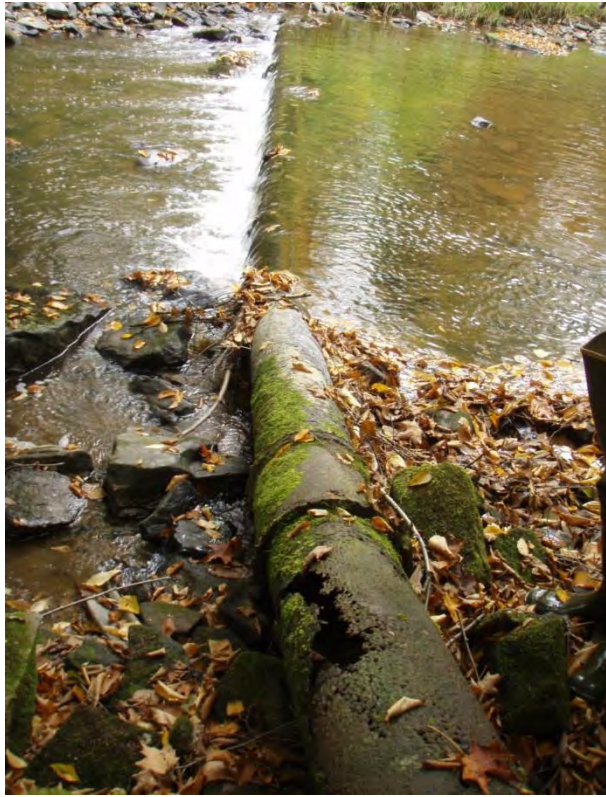
5963: Old, inactive metal pipe creating a potential AOP barrier, as well as safety hazard.
