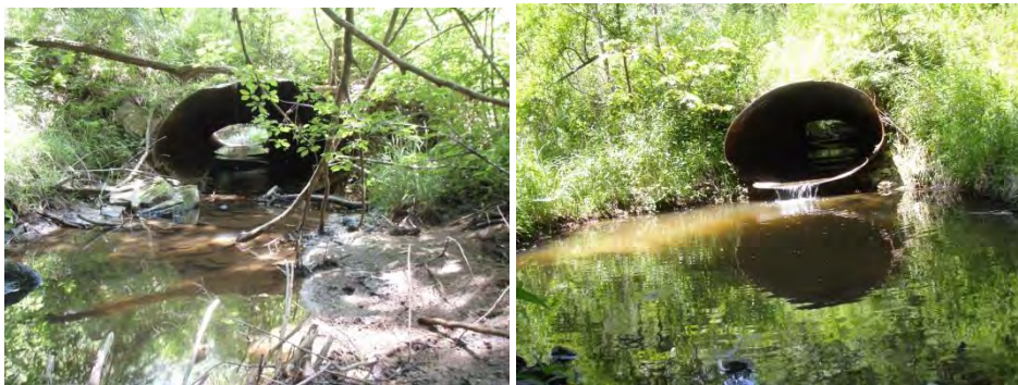
5966: Culvert inlet (left) and perched outlet (right) with scour pool.
