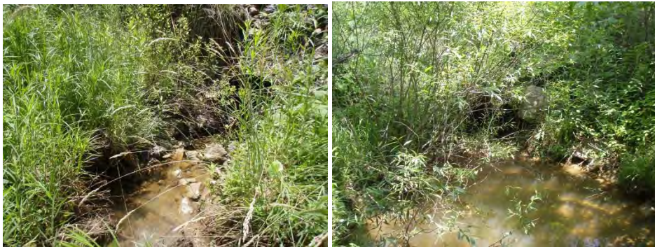
5965: Undersized culvert inlet (left) and outlet with scour pool (right).
