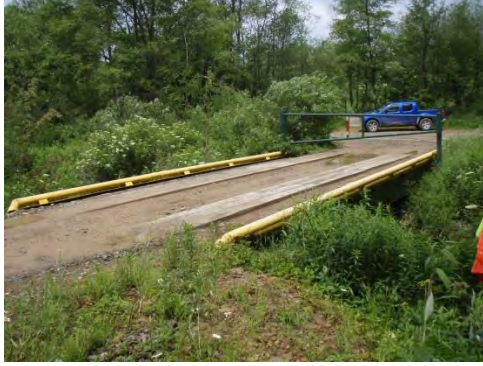
6045: Bridge causes slight constriction at high flows, but has good floodplain development beneath. Low potential for AOP barrier.
