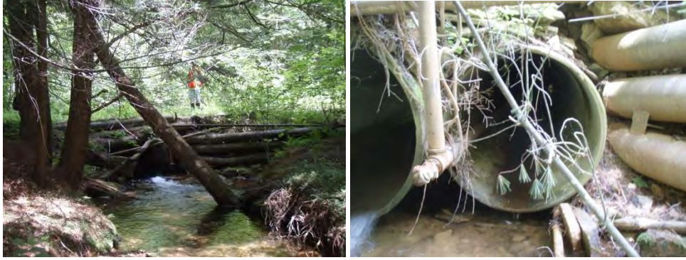
6034: Perched culverts on Rock Run (left), with 1 culvert containing an active 2" natural gas line (right).
