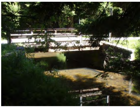
6141: Potential AOP barrier due to narrowness and lack of floodplain beneath bridge.
