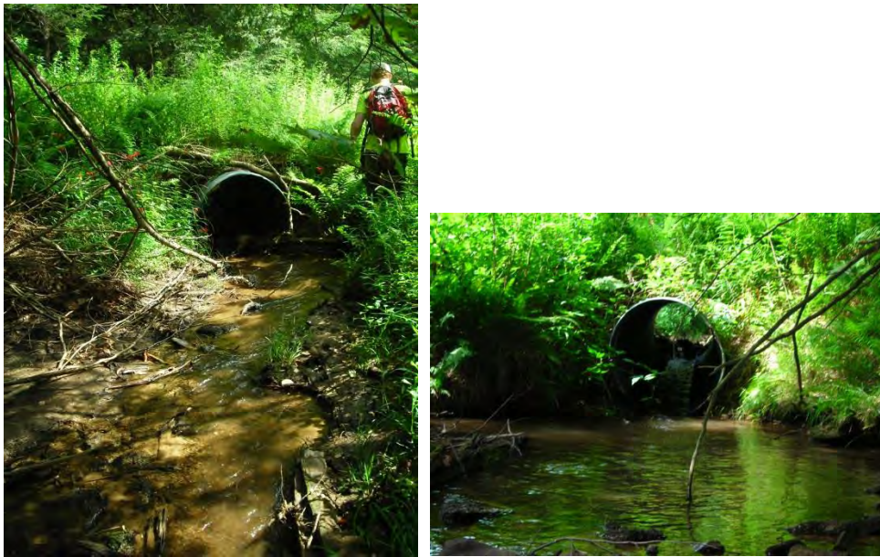
6035: Culvert perched, lacking substrate.
