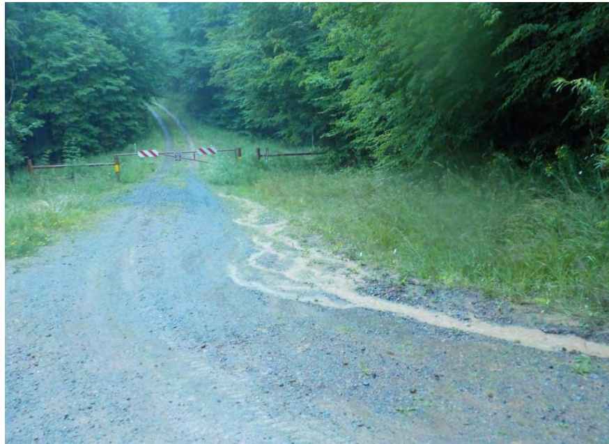
5806: Poorly maintained dirt and gravel roads throughout this and other drainages contributed sediment during heavy precipitation or runoff events, at times even preventing accurate assessments (and thus a canceled field day).
