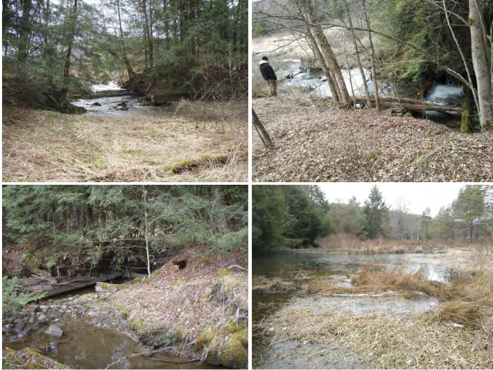
6234: Clockwise from top left: breached dam, timbers of dam structure, beaver ponds in relic impoundment, secondary breach. This breached dam creates a partial AOP barrier.
