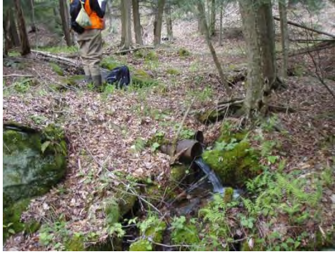
5978: Perched culvert outlet, 1 of 3 channels on this UNT at this inactive pipeline crossing.
