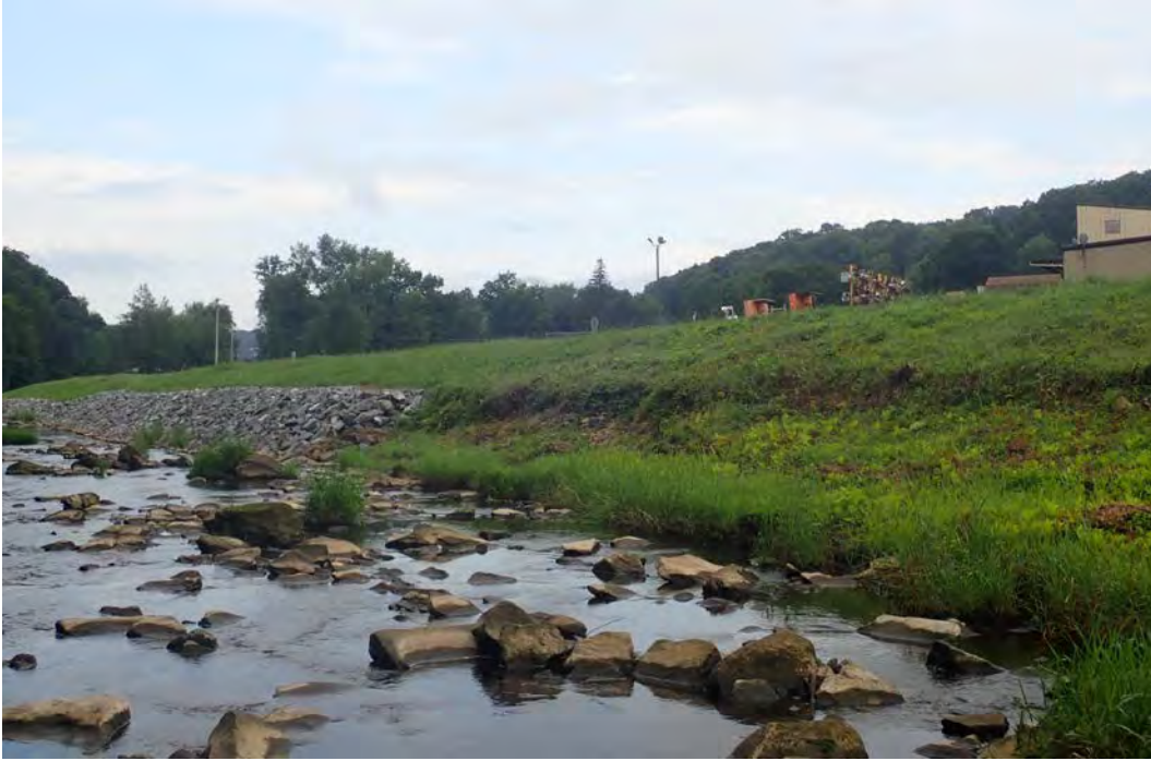
Photo 144. Right bank erosion and riprap bank stabilization near the PennDOT building.
