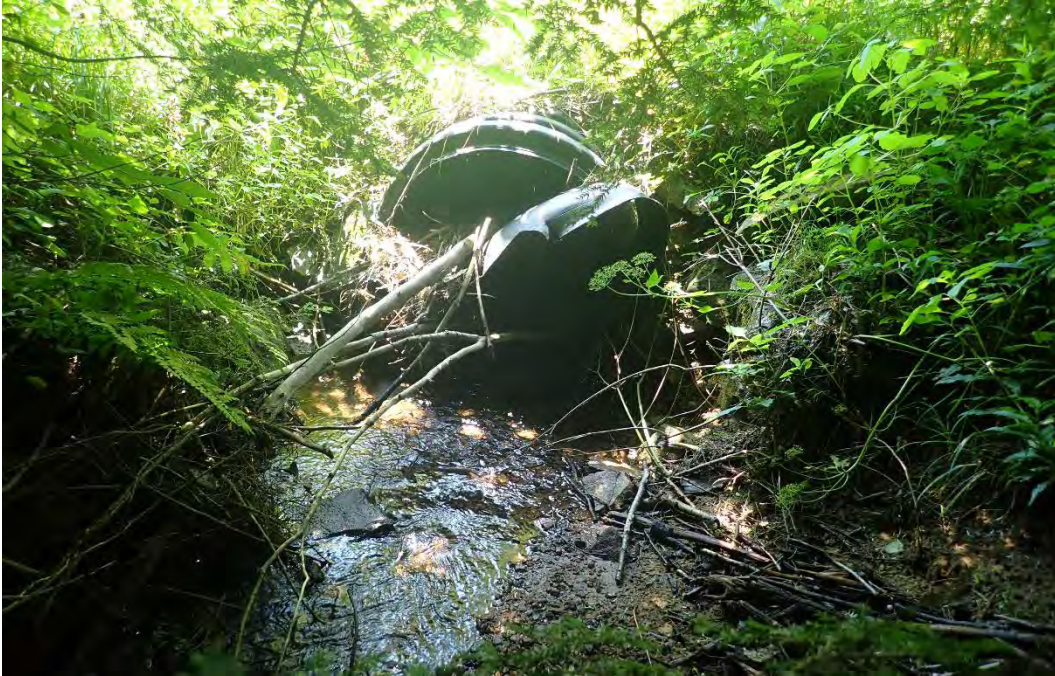
Photo 5. Clogged culvert inlet under a driveway along Windfall Road in EC04. Replacing the culvert with a larger structure would allow debris and aquatic organisms to pass through, as well as prevent flood waters from overtopping the driveway.
