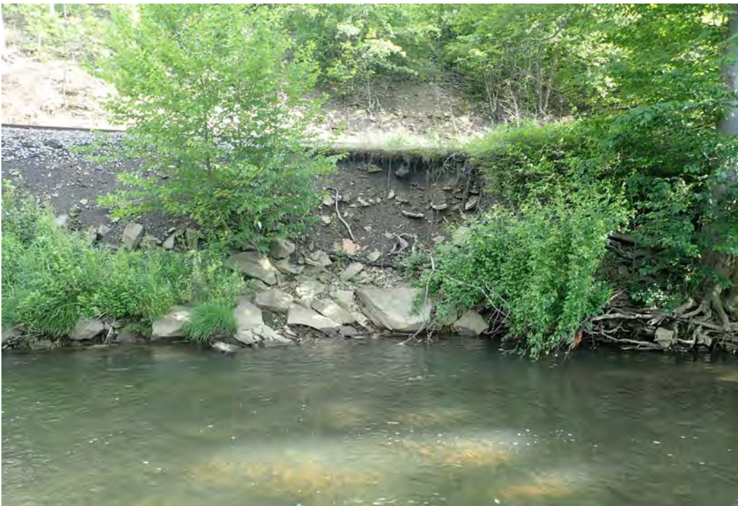
Photo 69. Erosion along the railroad in EC02. Installing streambank stabilization structures would help prevent further erosion.
