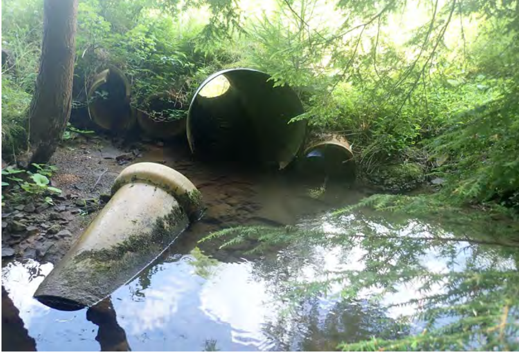
Photo 7. Culvert outlet under a driveway off of Windfall Road in EC04 with multiple, undersized pipes.
