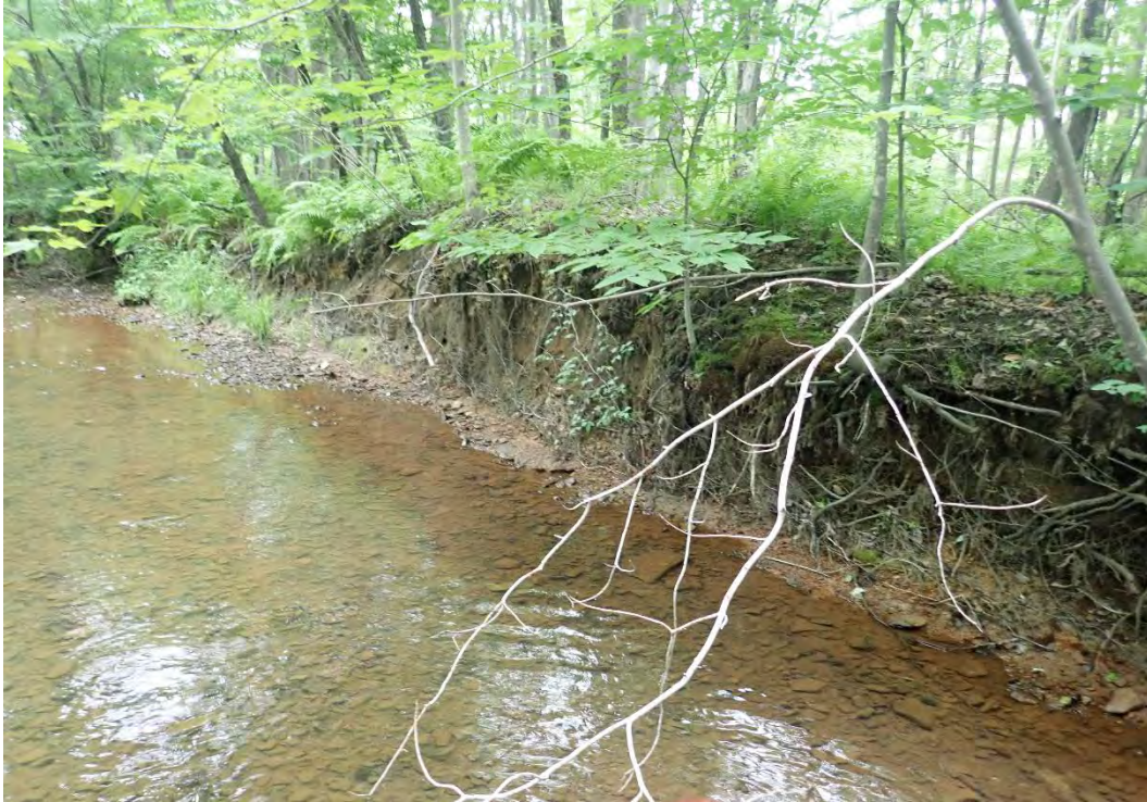
Photo 12. Eroded left bank in EC03.
