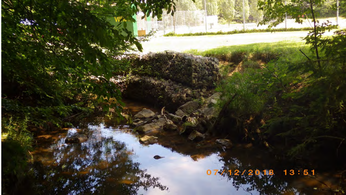
Photo 3. Looking upstream at gabion baskets along the streambank in Benzinger Park. The stream eroded the right bank near a paved walking trail. The gabion baskets were in poor condition and had protruding wires and were losing rocks to the stream.
