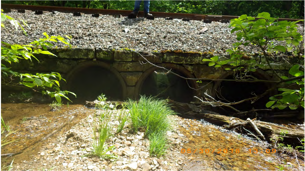
Photo 5. Inlet of railroad culvert. Sediment aggraded before the inlet, due to multiple, undersized culvert pipes which created a depositional area. The drop from the streambed to the bottom of the culvert pipes was estimated to be 1 foot high.
