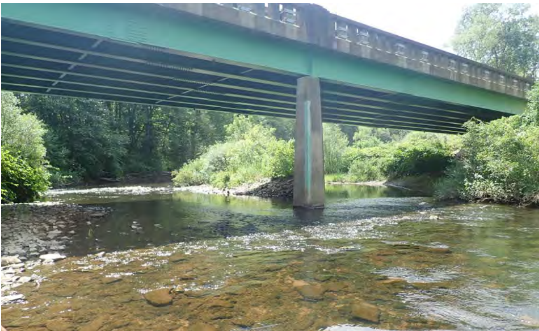
Photo 121. Looking downstream at the Highway 120 bridge over EC17. A gravel bar has formed behind the center abutment.
