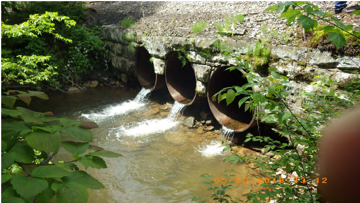
Photo 6. Outlet of railroad culvert in Photo 5. The drop from the middle pipe to the stream bottom was estimated to be 1 foot high. The inlet and outlet drops, in addition to the low water volume through the pipes, are barriers for aquatic organism p
