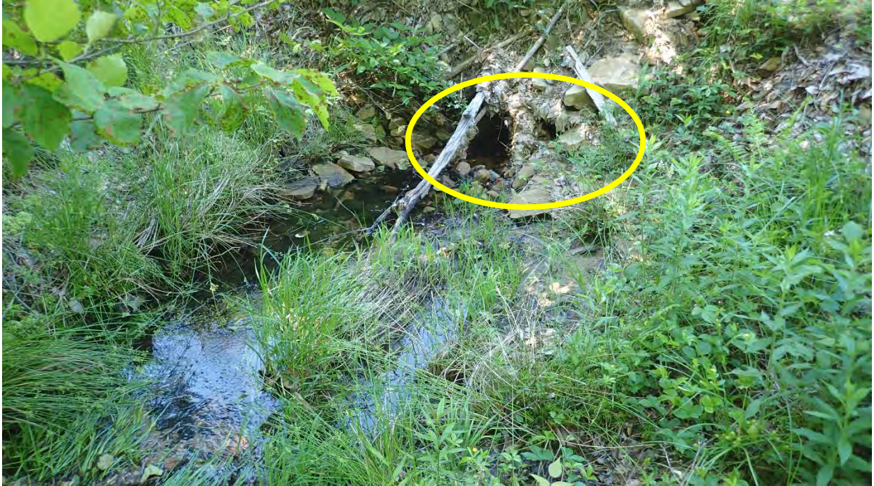
Photo 3. Beginning of Decker Run and clogged culvert pipes. A pool formed behind the pipes (yellow circle) due to debris and sediment aggradation.
