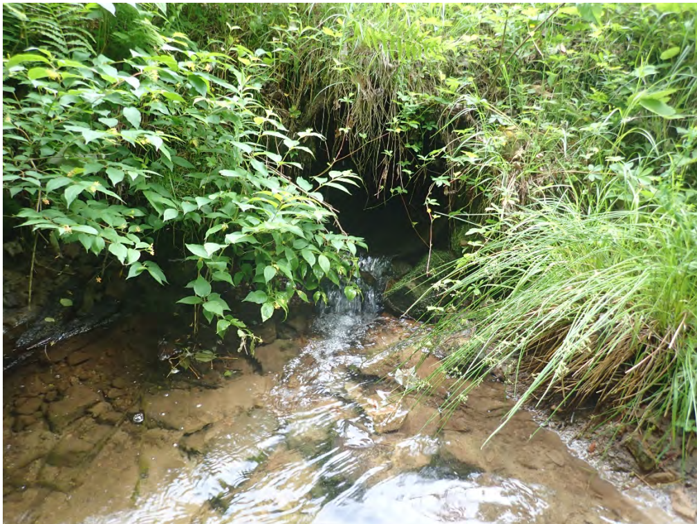
Photo 6. Outlet of the culvert from Photo 5. The outlet is perched about 8 inches from the stream bottom and could present an aquatic organism passage issue.
