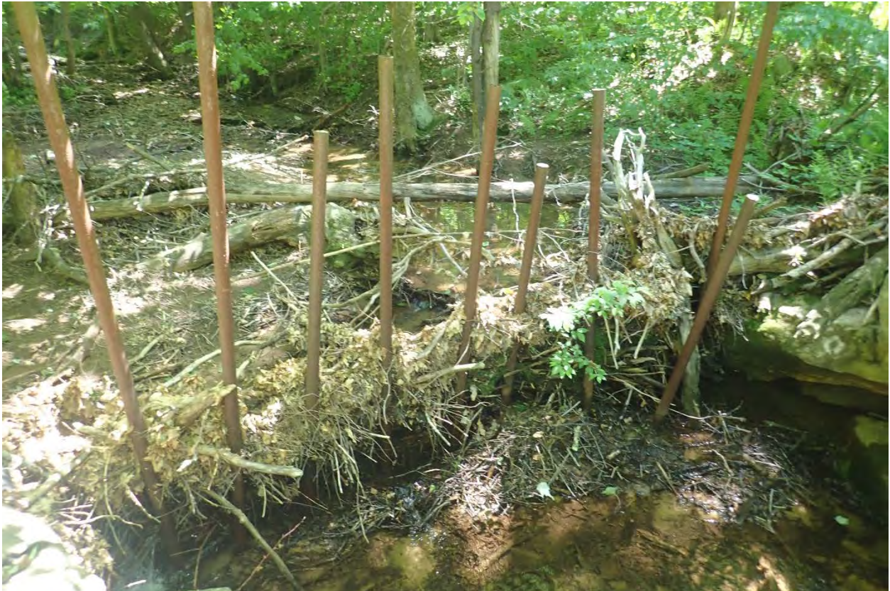
Photo 2. Inlet of the culvert from photo 1. Vertical metal pipes blocked debris from entering the culvert pipes, but created a large sediment bar upstream.
