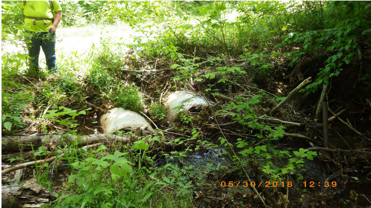
Photo 1. Inlet of triple culvert underneath gravel road. The culverts did not have the capacity to allow woody and inorganic debris to pass downstream and collect debris at the inlet. The debris, in this instance, created a barrier for water, debris, and aquatic organisms to pass.
