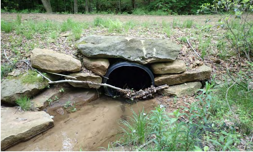
Photo 2. Inlet of PA Game Commission dirt road culvert. The inlet drops about 6 inches from the stream bottom, which has aggraded, to the bottom of the pipe.
