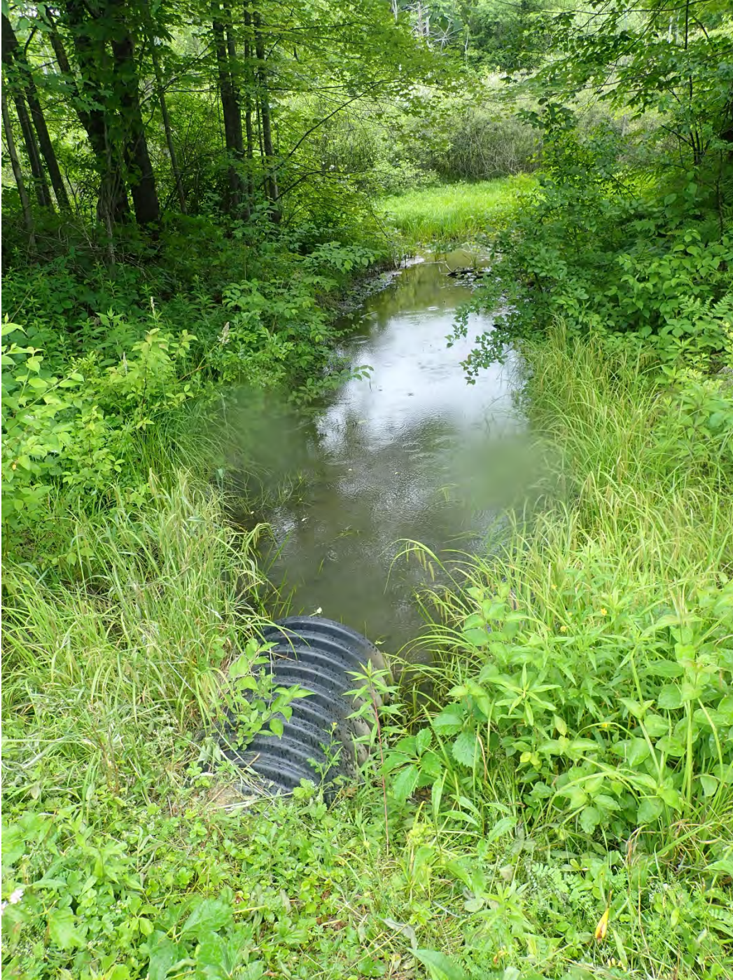
Photo 3. Culvert at the end of TC02 beneath Joseph Road. The culvert was undersized. From the dirt residue on the pipe, it is obvious that the stream overtops the culvert during high flow. Aquatic organisms, greater water volume, and material could pass more efficiently through the culvert if it were to be replaced with an appropriately-sized structure.
