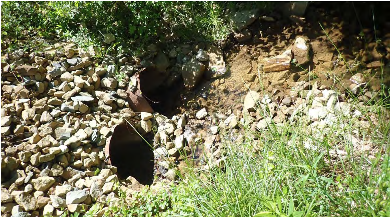
Photo 4. Outlet of the pipes from photo 3. The majority of stream flow routes through the pipe closest to the left bank due to debris jams at the inlet.
