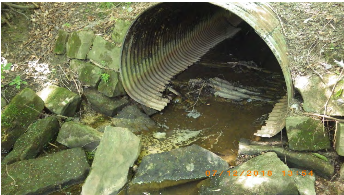
Photo 4. Culvert outlet in poor physical condition on the unnamed tributary to IR01 through Benzinger Park. The culvert was a barrier to fish passage during assessment due to low flow.
