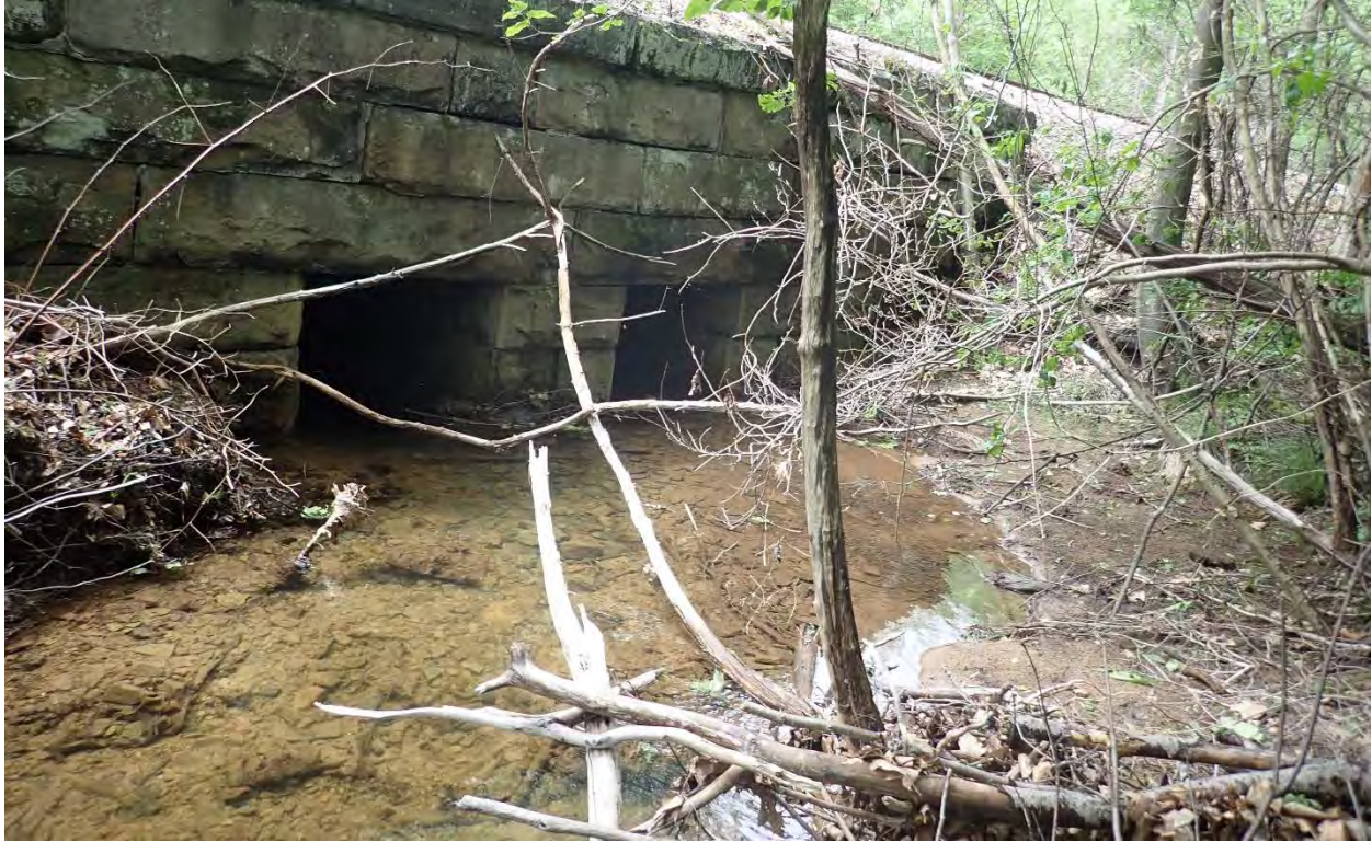
Photo 5. Inlet to the railroad culvert. The undersized, misaligned culvert collects sediment and debris at the inlet causing stream bed aggradation and creating a 1ft high inlet drop.
