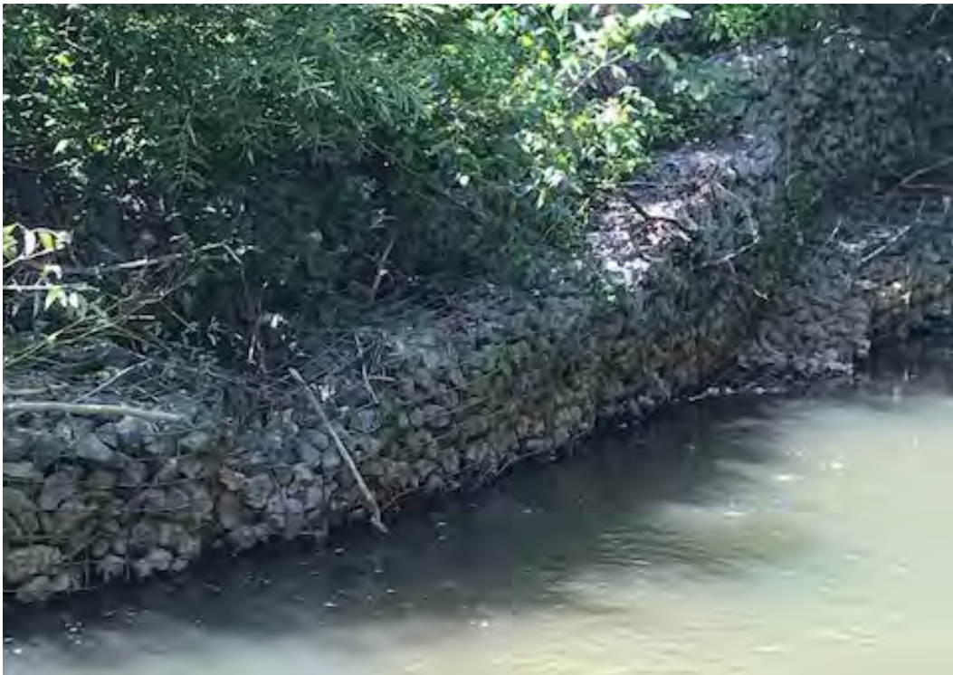
Photo 49. Slumping gabion baskets in EC10. Gabion baskets often fail over time and provide no habitat for aquatic organisms. Damaged basket wires can be an injury hazard.
