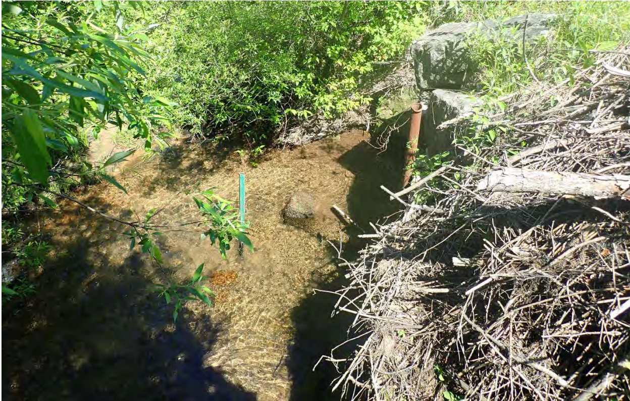
Photo 6. Looking down at the inlet of the railroad culvert. Stakes were placed at the inlet to prevent woody debris from entering and passing through the culvert. Though there was no debris jam observed during assessment, it was evident that debris collects at this point and is removed regularly (likely by the railroad) due to deposition and a drop to the pipe inlet.
