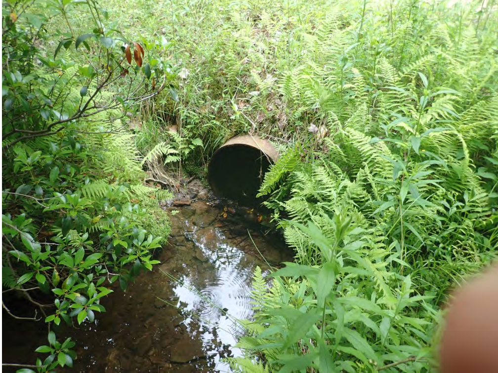
Photo 5. Culvert inlet in LR02. Culvert goes beneath Laurel Run Road on Saint Marys Water Authority Property.
