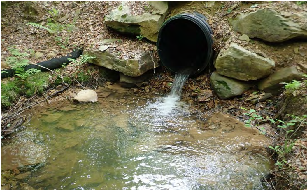
Photo 3. Outlet of the same culvert from photo 2. The outlet drops about 8 inches from the bottom of the pipe to the bottom of the stream. A lack of substrate in the pipe, as well as fast and shallow flow, could create aquatic organism passage issues at low flow.
