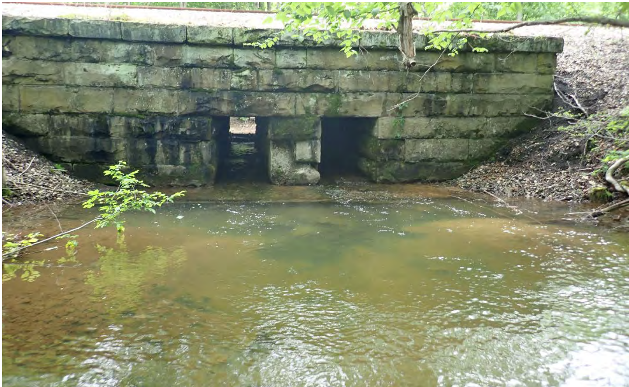
Photo 6. Railroad culvert outlet. The structure has shallow water depth and likely dries during periods of low flow.
