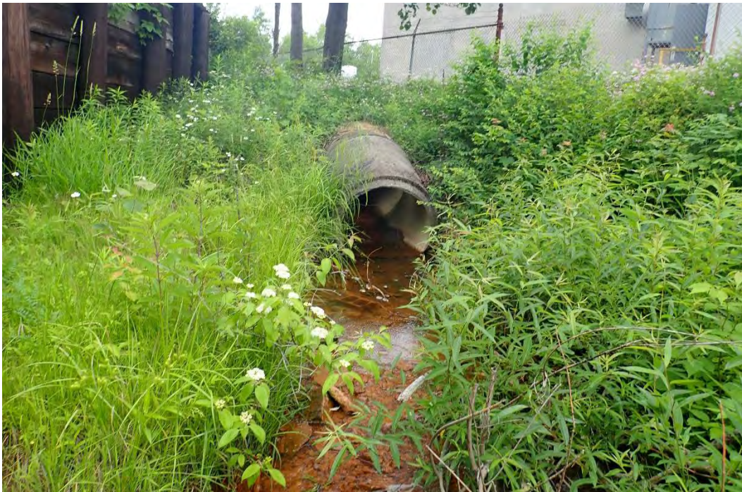
Photo 17. A drain near Enhanced Sintered Products discharging red water into EC03. Specific conductivity of the discharged water was elevated at 300 \mu\text{S}/\text{cm} .
