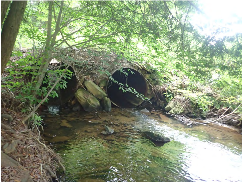
Photo 16. Culvert outlet from photo 16. The left pipe is slightly perched and flow is low in both pipes.
