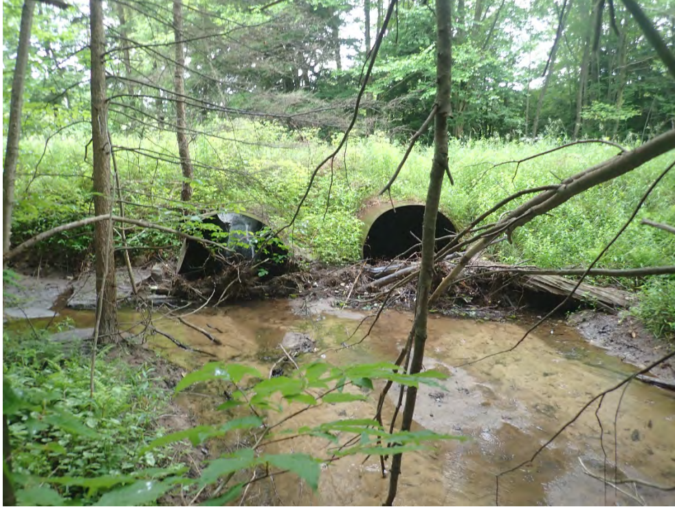
Photo 15. Culvert inlet in section LR03 created a sand bar and debris jam that could make the culvert unnavigable for aquatic organisms. Culvert goes under a decommissioned section of the Million Dollar Highway.
