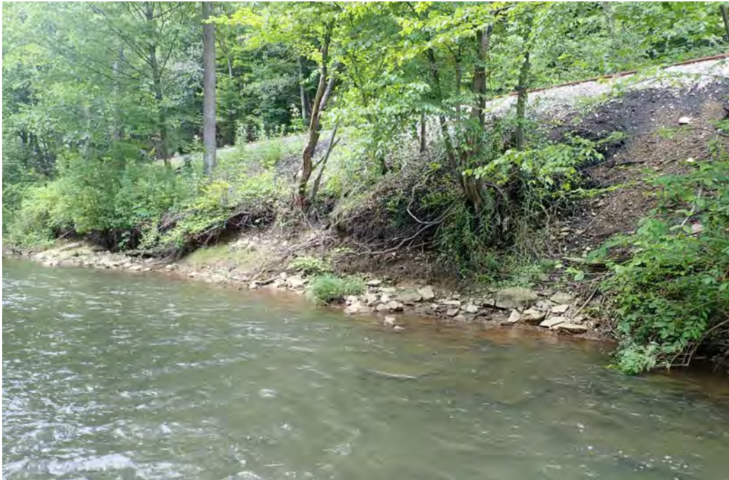
Photo 96. Right bank erosion along the railroad bed in EC08.
