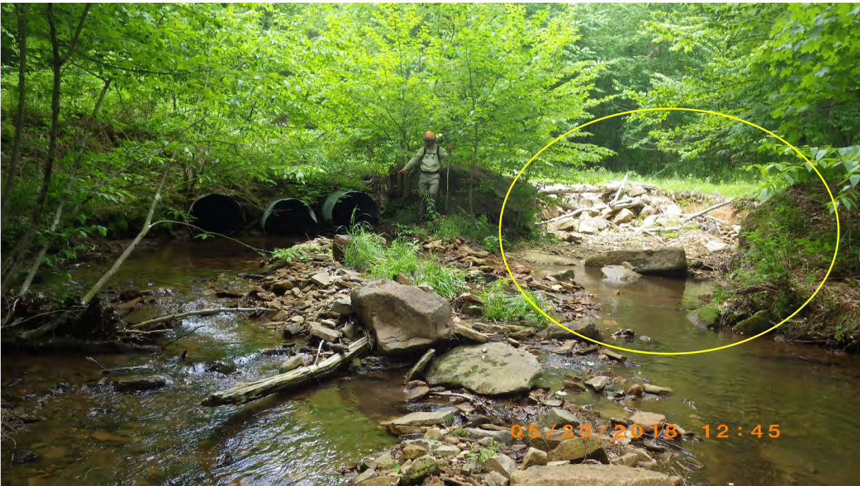
Photo 2. Outlet of the triple culvert in Photo 1. The gravel road was eroding into the stream within the yellow circle. The undersized culvert caused water to pool, route around the stream crossing, and flow back into the stream at the circled location. The erosion was secured with rip-rap, though erosion continued to actively occur.
