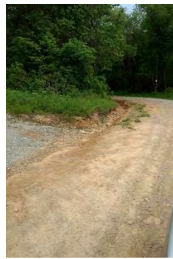
Greenlick Hollow Road – dirt and erosion
