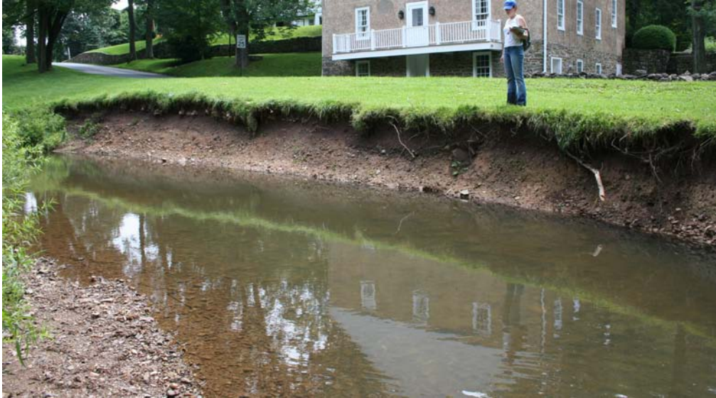
Figure 12. This severely eroded streambank is adding sediments to the overall creek system and could jeopardize the nearby roadway if erosion is not controlled. Restoration of this section of the Hosensack Creek could be a prominent demonstration project.
