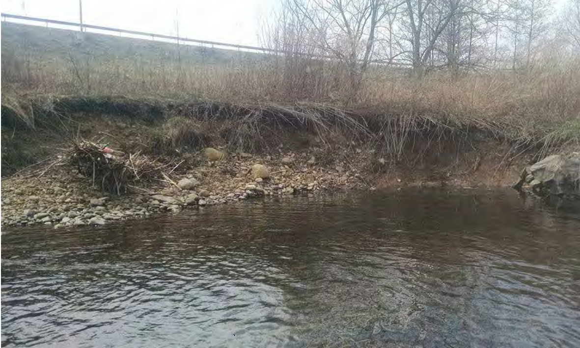
Figure 17: Erosion Near LR4 (Photo 12)
