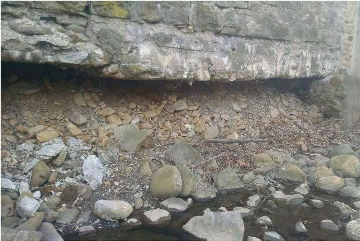
Figure 18: Flood Wall Undercutting (Photo 13)
