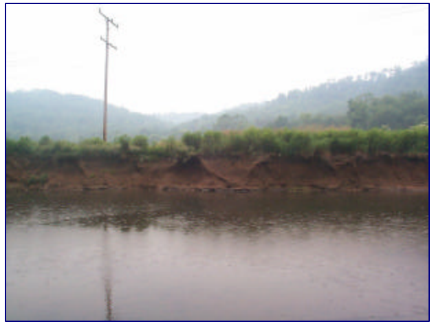
Erosion along the bank of Mill Creek.
