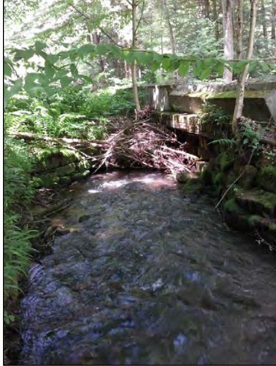
Barrier 3: illustrates how undersized culverts collect flood debris; adequately-sized culverts pass debris of this size, and much larger, more easily
