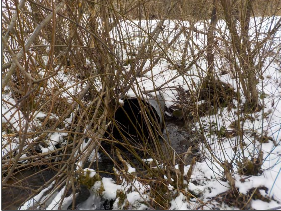
Barrier 10 is located on a vegetated road that provides access for PGC to manage food plots located in this area. Due to the minimal amount of traffic this crossing receives, a stable ford is recommended to replace this undersized culvert.
