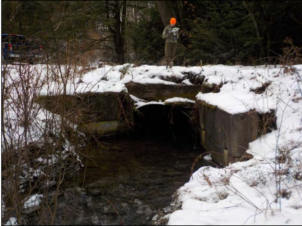
Barrier 8 outlet: some stream substrate is present through the crossing, making this barrier one of the more passable crossings in the watershed
