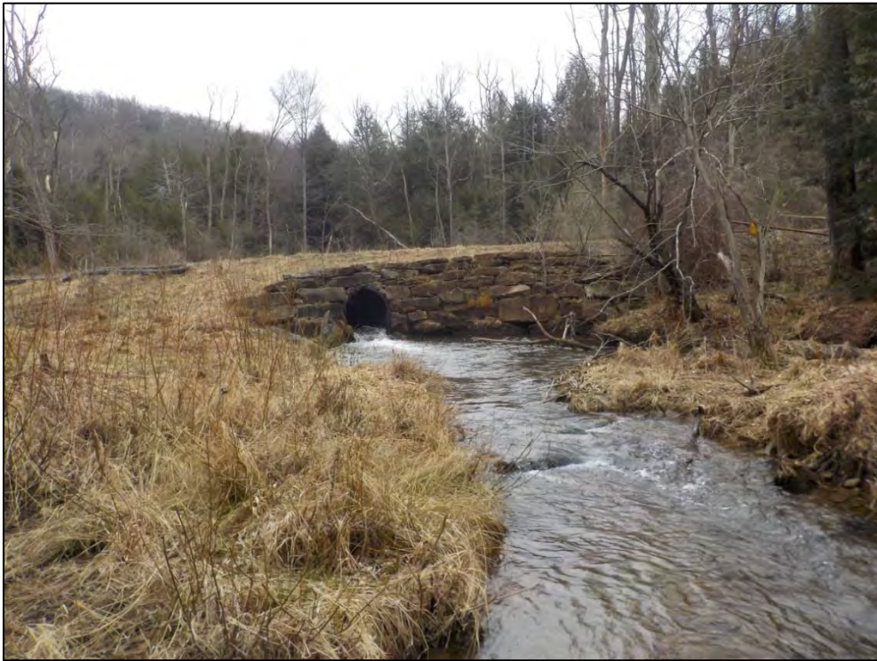
Barrier 7: a perched high-density polyethylene (HDPE) pipe with a smooth bore is a complete passage barrier. Access roads to both sides of the valley are present on the ridges. This passage barrier is recommended to be removed and the stream and floodplain fully restored.
