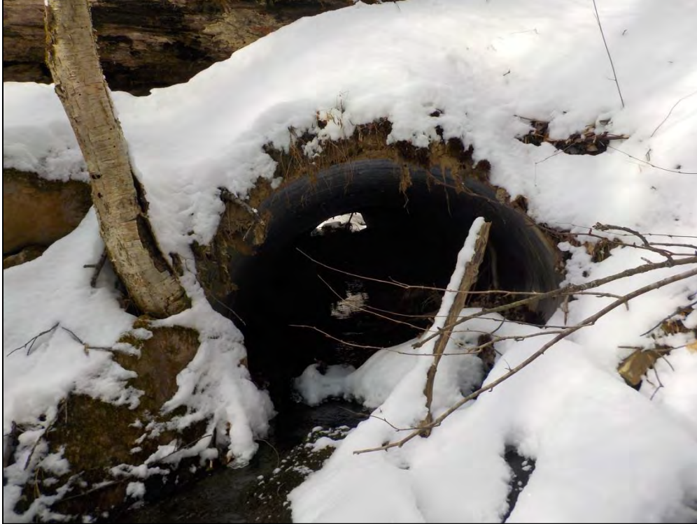
Barrier 12: squash pipe outlet on segment 5A1-Meyers Hollow; this culvert is rusted through portions of the bottom
