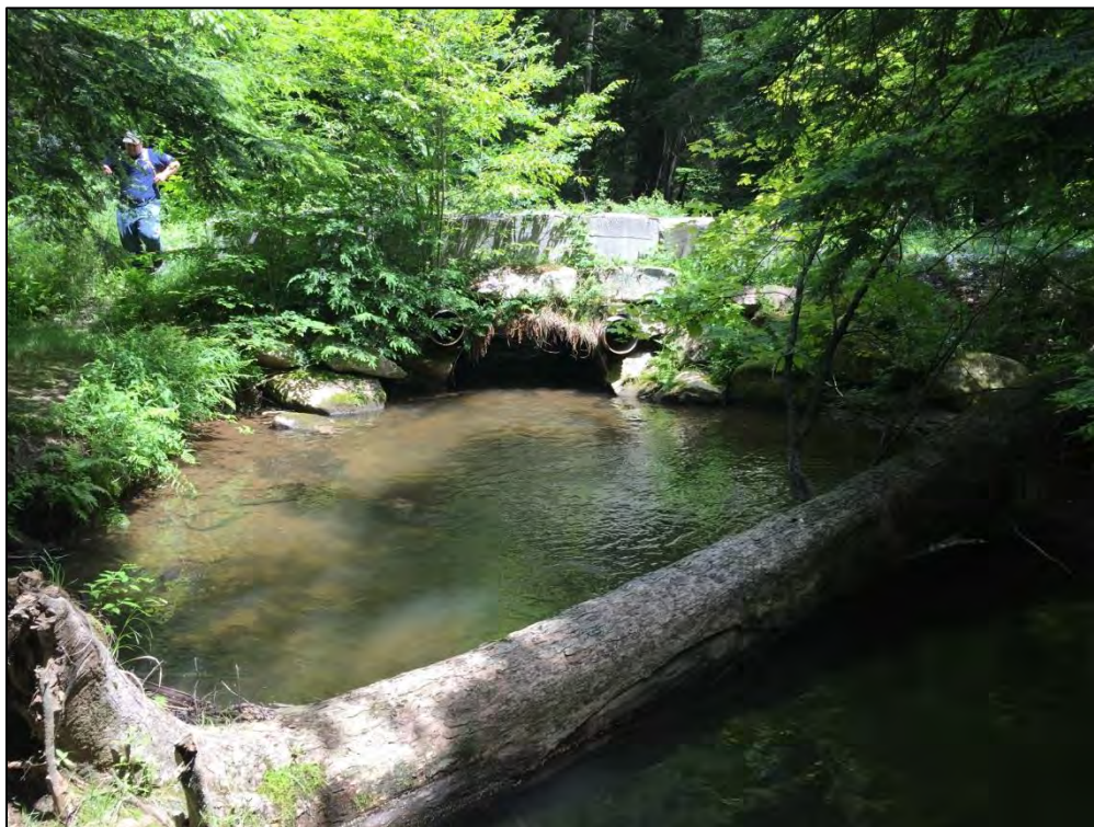
Barrier 2 Outlet: note the size of the scour pool compared to the culvert
