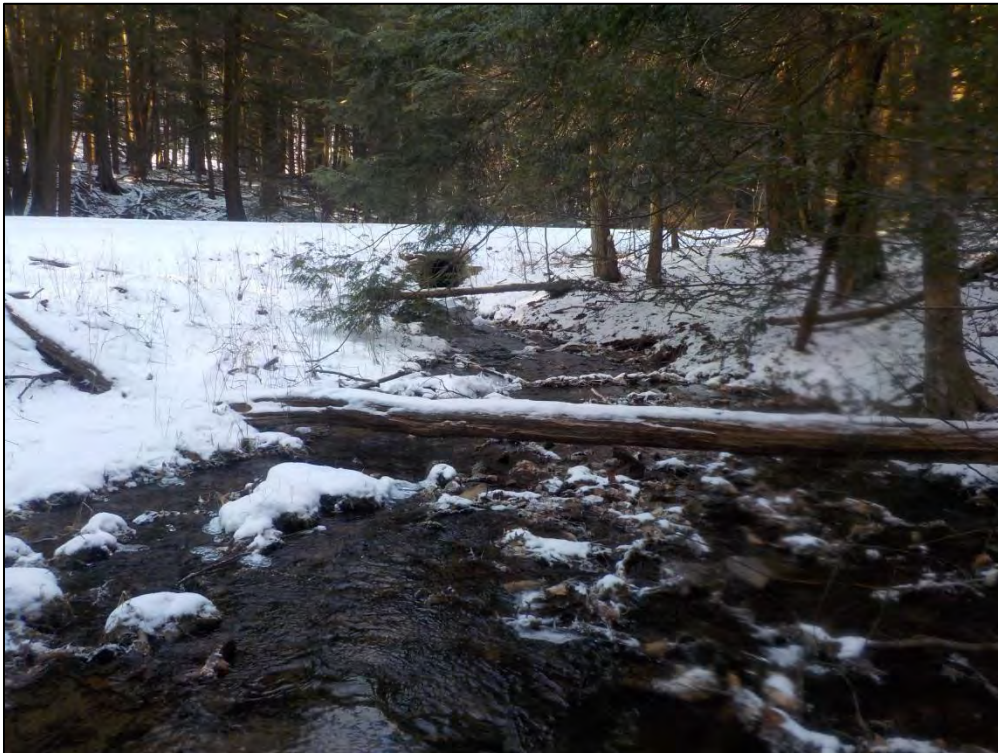
Barrier 11 outlet: Located on segment 8, this HDPE pipe has a smooth bore and, due to high velocities in the pipe, prevents aquatic organisms from migrating upstream.
