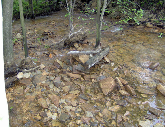
Cobbles and sediment below culvert shown above.
