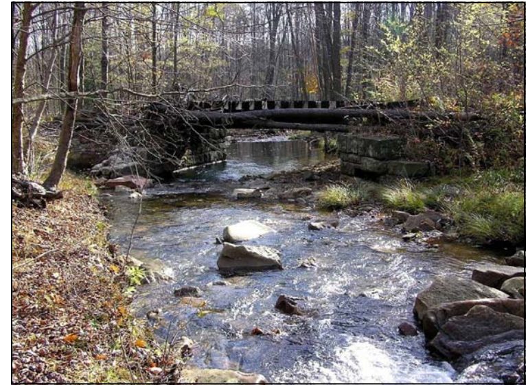
A bridge, no longer used by trains, spans Bear Run at BR-3.
