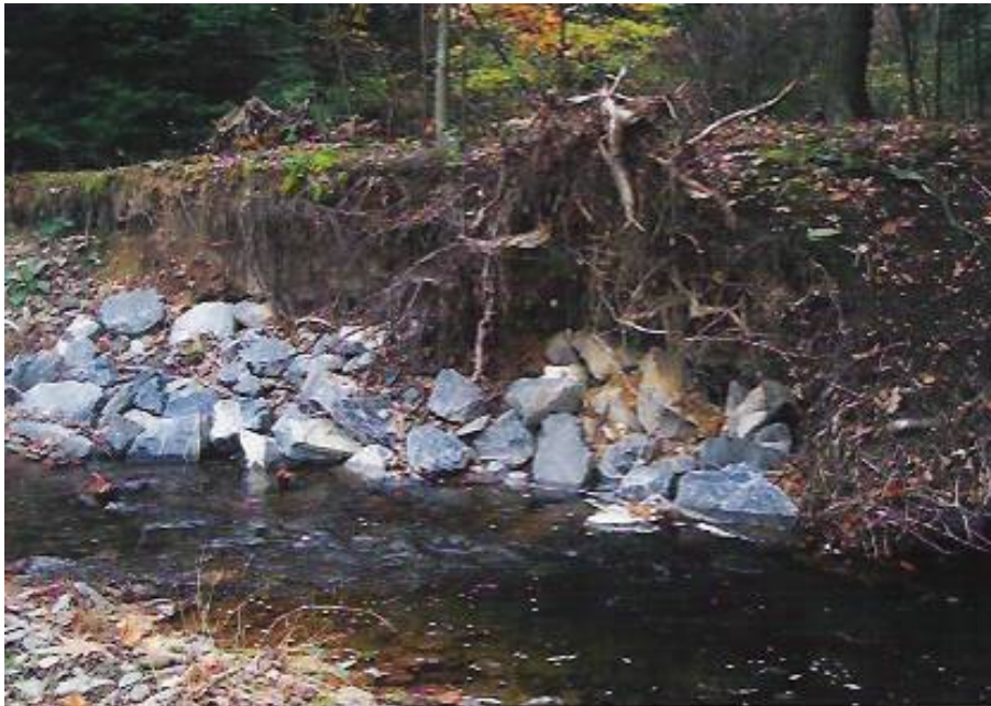
Mugser Run 3 (MURU3). Note unstable bank and failed riprap project. Photo by Winnie McNelis.
