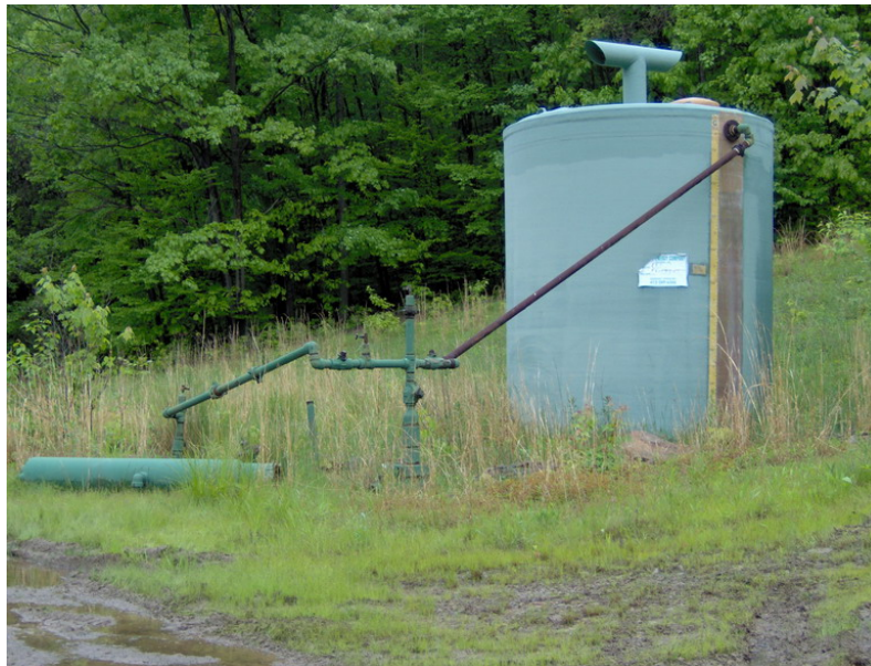
Gas well located along Bad Tributary
