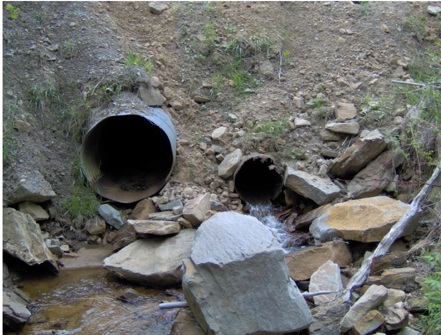
Culvert pipes under Rock Run Road. Note the lack of vegetation to stabilize area.
