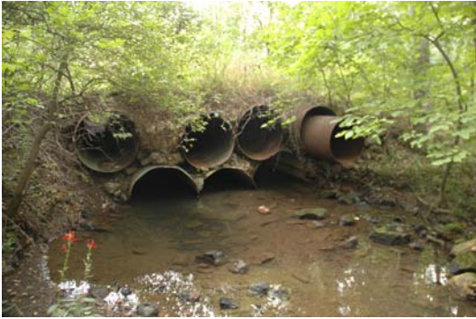
Figure 17 Shobers Run Lane crossing and sediment-laden stream channel
