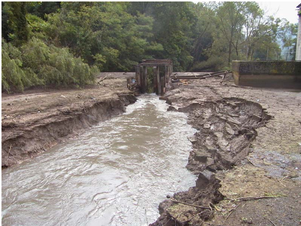
Photo 4: Newly eroded channel upstream of Reedsville Milling Company Dam.
