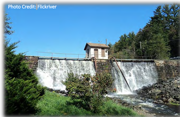
Figure 13. Overflow from the Huntsville Dam in the Huntsville Creek subwatershed of larger Toby Creek Watershed 36
