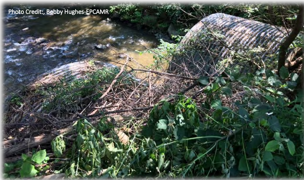
Figure 11. Double Metal Corrugated Squashed Pipes directing flow of Toby Creek under State Route 309 adjacent to the DAMA
