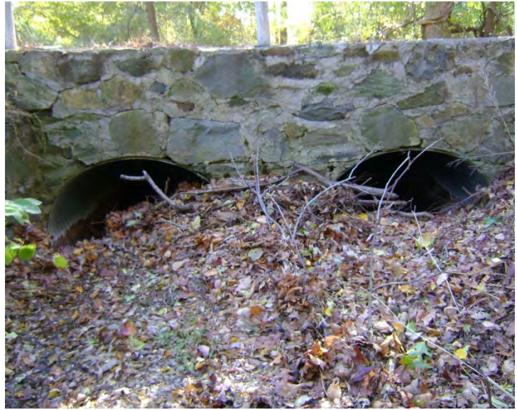
Figure 20. Debris blocking Forest Lane culvert intake.
