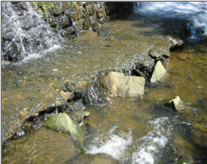
Figure 7. Scour downstream of the concrete footing.
