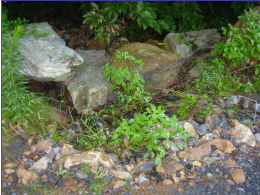
Figure 8. Recent scour and gully formation along the eastern flank of the dam structure
