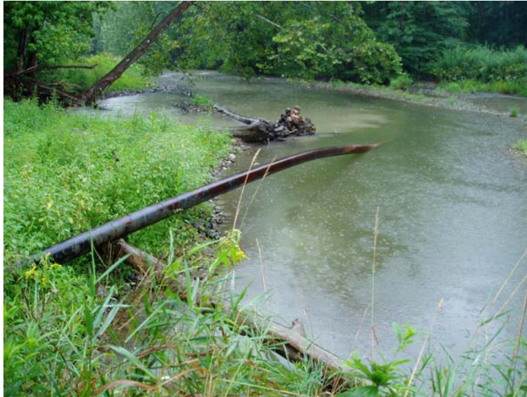
Figure 19. Exposed pipe at the confluence of Wallace Run and Bald Eagle Creek
