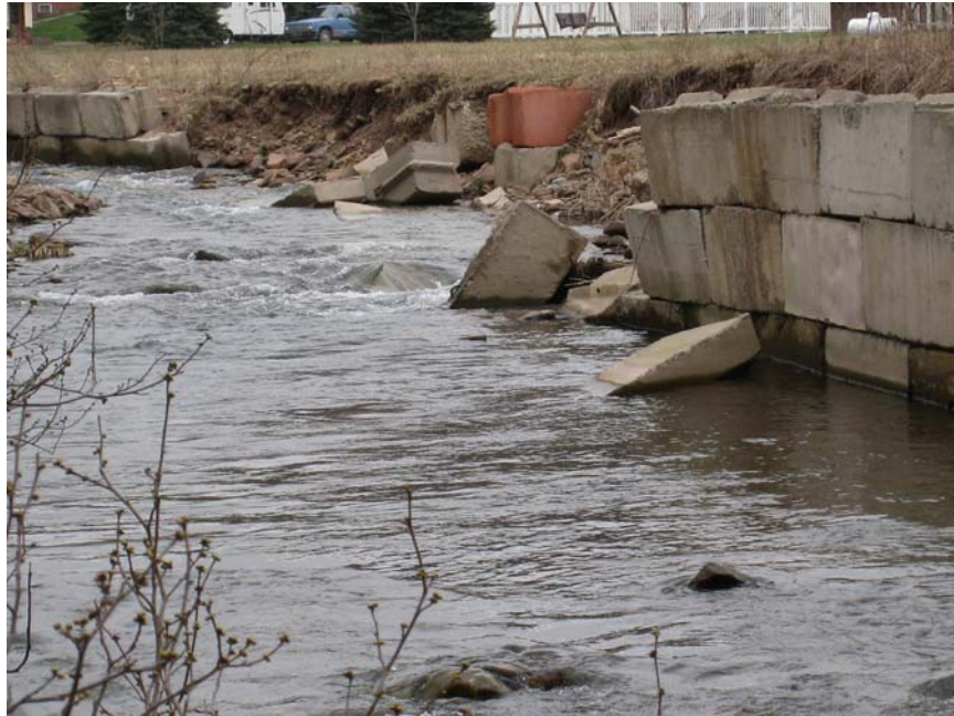
Figure 6. Even large concrete blocks were not sufficient to stabilize the bank.
