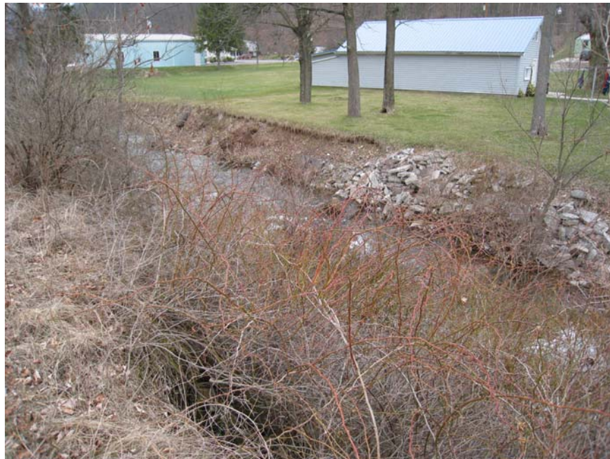
Figure 5. Homes and businesses border the lower four miles of Wallace Run. Much of the riparian vegetation has been replaced with lawn, resulting in substantial bank erosion that needs continuous maintenance.
