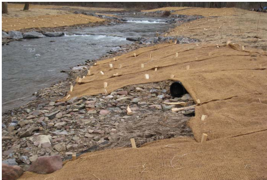
Figure 13. Jute matting stabilizes the bank until shrub plantings develop, and cross veins scour deep pools to provide habitat for trout.
