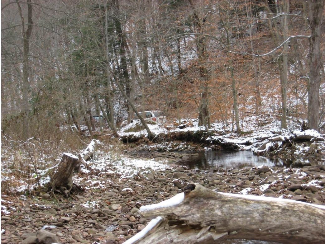
Before picture of eroding streambank along Bobs Creek in Blue Knob State Park.
