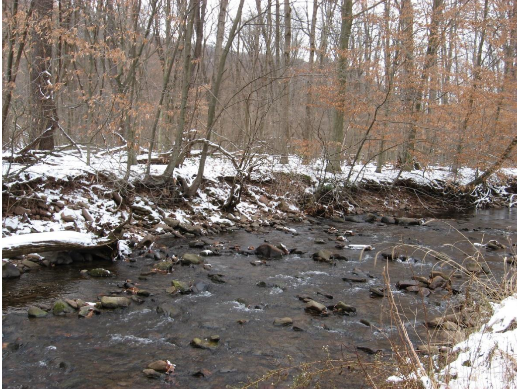
Before photo of eroding streambank along Bobs Creek in Blue Knob State Park.
