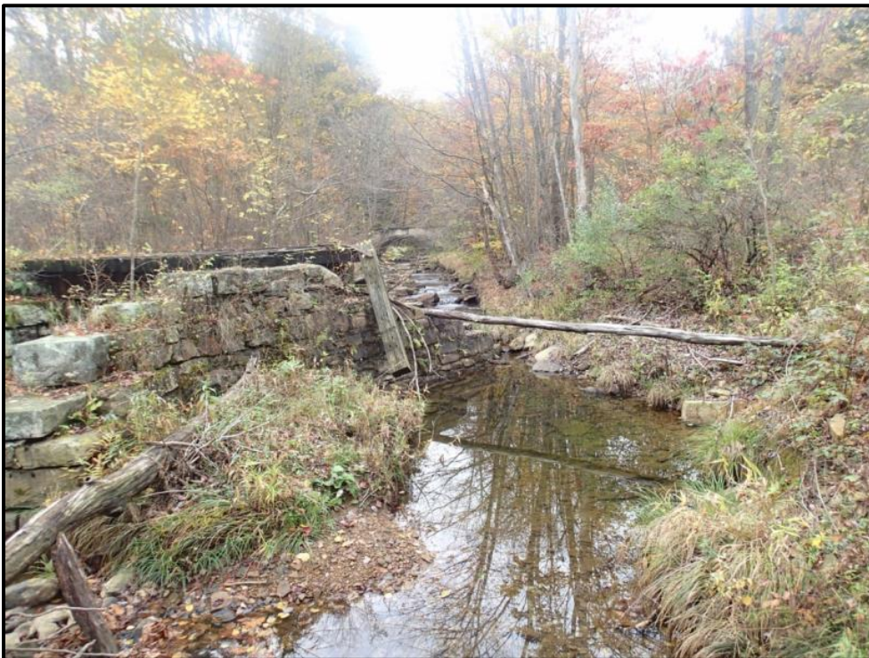
Figure 4 depicts the bridge pier that was removed as well as the eroding bank that was addressed by our project.
