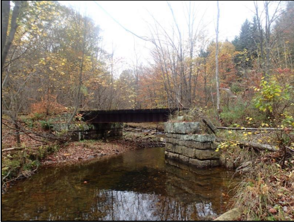
Figure 3 is the abandoned railroad bridge. This perspective is looking upstream from the confluence of the North and South Branches of Bear Run. The unstable, eroding streambank is to the right of this photograph.
