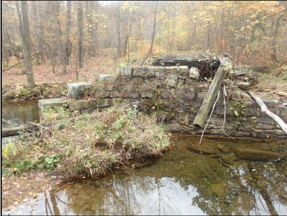
Figure 5 shows the collapsing bridge pier from the perspective of standing on the eroding bank.
