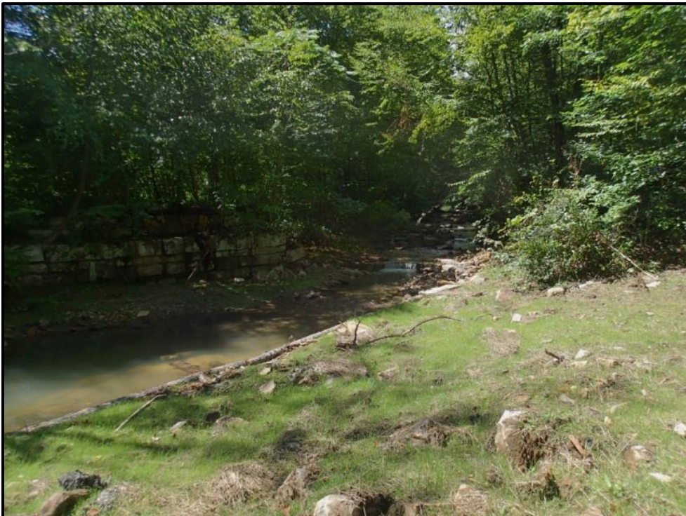
Figure 10 - View of the mud sill and cross vane one month after project completion
