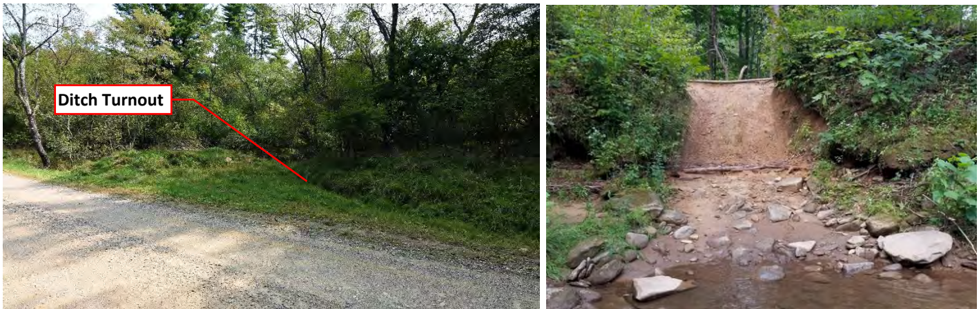
Figure 31. Ditch turnout into Woodcock Run on Pike Road (photo left) and ATV crossing on Pithole Creek mainstem near mouth at Oleopolis (photo right).
