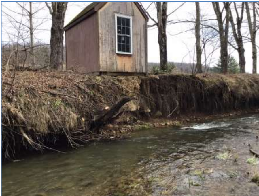
FIGURE 14 – BANK EROSION NEAR PRIVATE POND ALONG SOUTH FORK
