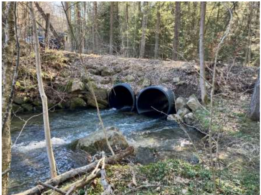
FIGURE 7 - A MULTI PIPE CROSSING ON MILL CREEK RESTRICTS AOP
