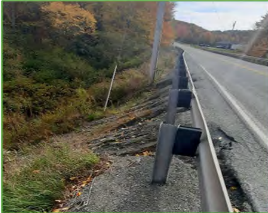
Figure 8 Sedimentation source at 171 Bridge location
