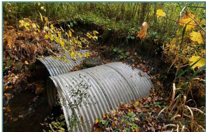
Figure 15 Crossing 92241 Culvert pipe with eroded surrounding crossing base
