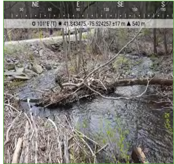
Figure 28 Ogden Road culvert causing stream to back up and erode new channel
