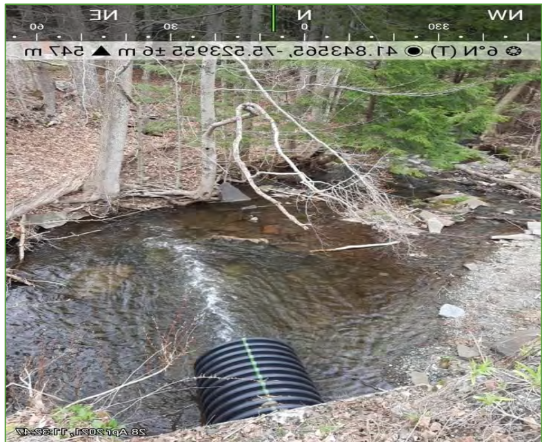
Figure 18 Crossing 89679 at Ogden Road with scour pool
